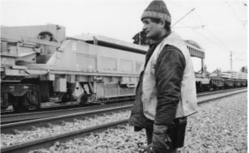
Poland: 2.5 kilometres of track a day, thanks to the automated track-laying train from Switzerland.
