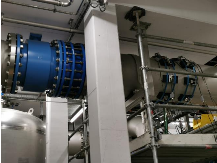
On-Site Verification of a MAG-Meter
