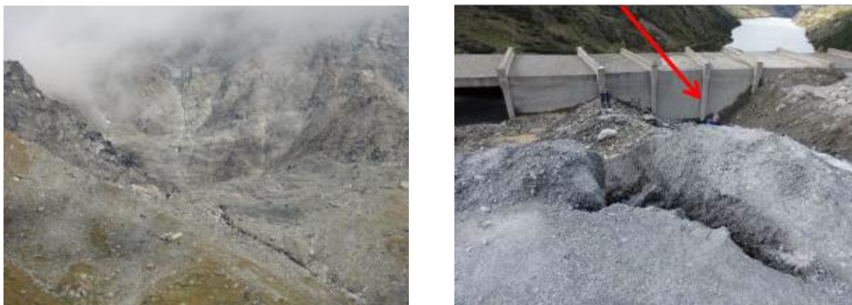
Figure 11, left: Zone visible from the road, located just below the source of the hazard. Right: Protection gallery showing the section fortified with reinforced concrete (red arrow) and the masonry section that was destroyed.
